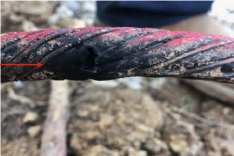
Faulted Direct buried #2 Al Cable with exposed concentric neutral
