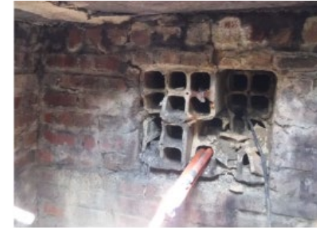
Clay tile duct bank in disrepair (still in use with existing fiber)
