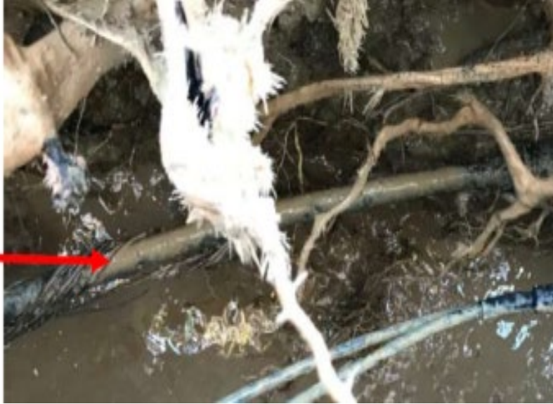
Exposed concentric neutral cable in ground with the neutral eroded away
