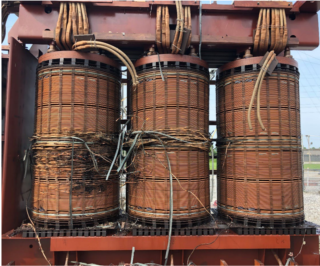
Transformer Failure (O'Fallon 21)
