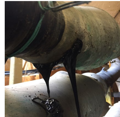
Abnormal PILC cable joints
