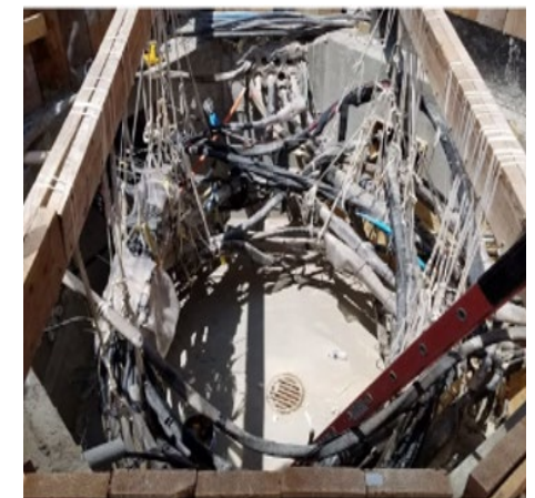
Highly congested manhole on 7 th St.
