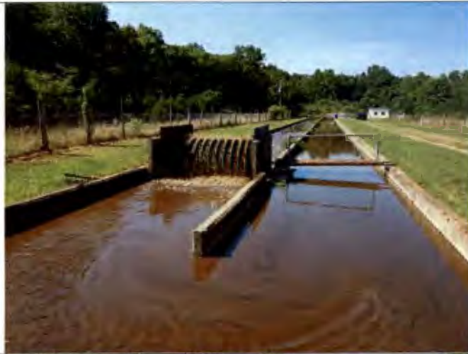
Photograph #: 001 Taken by: Wesley Hargraves Entity: Terre Du Lac Oxidation Ditch Permit: MO0095311 Location: St. Francois County Description: View of oxidation ditch and northern rotor. Taken facing south. Date Taken: July 10, 2019 Program: WPC Unit
