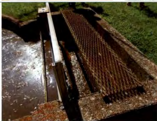
Photograph #: 003 Taken by: Wesley Hargraves Entity: Terre Du Lac Oxidation Ditch Permit: MO0095311 Location: St. Francois County Description: View of outlet box to clarifier. Taken facing southeast. Date Taken: July 10, 2019 Program: WPC Unit
