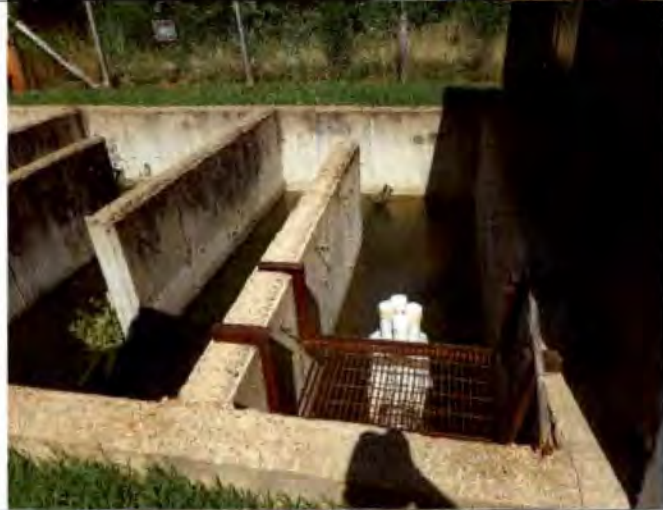
Photograph #: 005 Taken by: Wesley Hargraves Entity: Terre Du Lac Oxidation Ditch Permit: MO0095311 Location: St. Francois County
