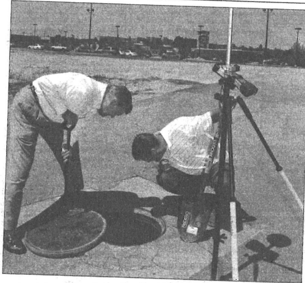
In this 2010 photo, Jon Fribis, right, and his father, Gene Fribis, check a sanitary sewer manhole in the Arnold Commons development. Their company's study turned up a number of problems in the city's aging sewer system.
