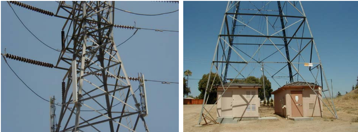
Cellular antennas and equipment sheds utilize transmission line towers.
