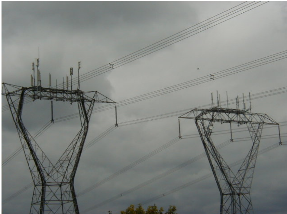
Communications and Cellular Antennas mounted on 500 kV transmission lines.
