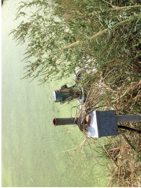
Mechanical Systems Failed
