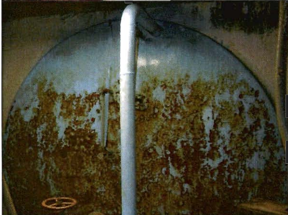
Photo #:4 Date Taken: 08/20/2014 By: Michelle Oglesby Program: PDWB File: Crawford County Location: Indian Hills Utilities Description: East end of 20,000 gallon ground storage, upper terminal.
