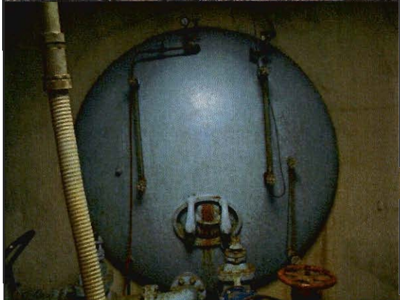
Photo #:7 Date Taken: 08/20/2014 By: Michelle Oglesby Program: PDWB File: Crawford County Location: Indian Hills Utilities Description: North end of 5,000 gallon pressure tank.
