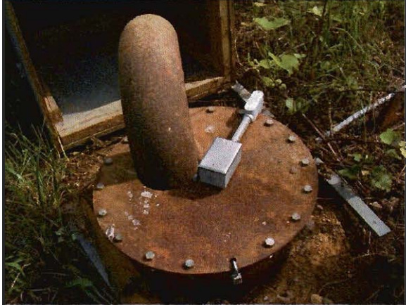
Photo #:6 Date Taken: 08/20/2014 By: Michelle Oglesby Program: PDWB File: Crawford County Location: Indian Hills Utilities Description: 20,000 gallon ground storage access hatch and vent/over flow piping.
