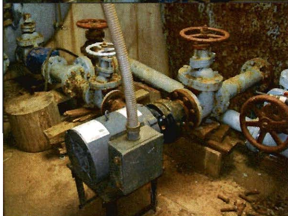
Photo #:8 Date Taken: 08/20/2014 By: Michelle Oglesby Program: PDWB File: Crawford County Location: Indian Hills Utilities Description: Pump and piping within the well house for Well #1.
