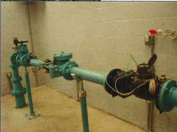
Photo #:012 Date Taken: 10/26/2016 By: Michelle Oglesby Program: PDWB File: Crawford County Location: Indian Hills Utilities Operating Co. Inc. Description: Well #3 - Piping
