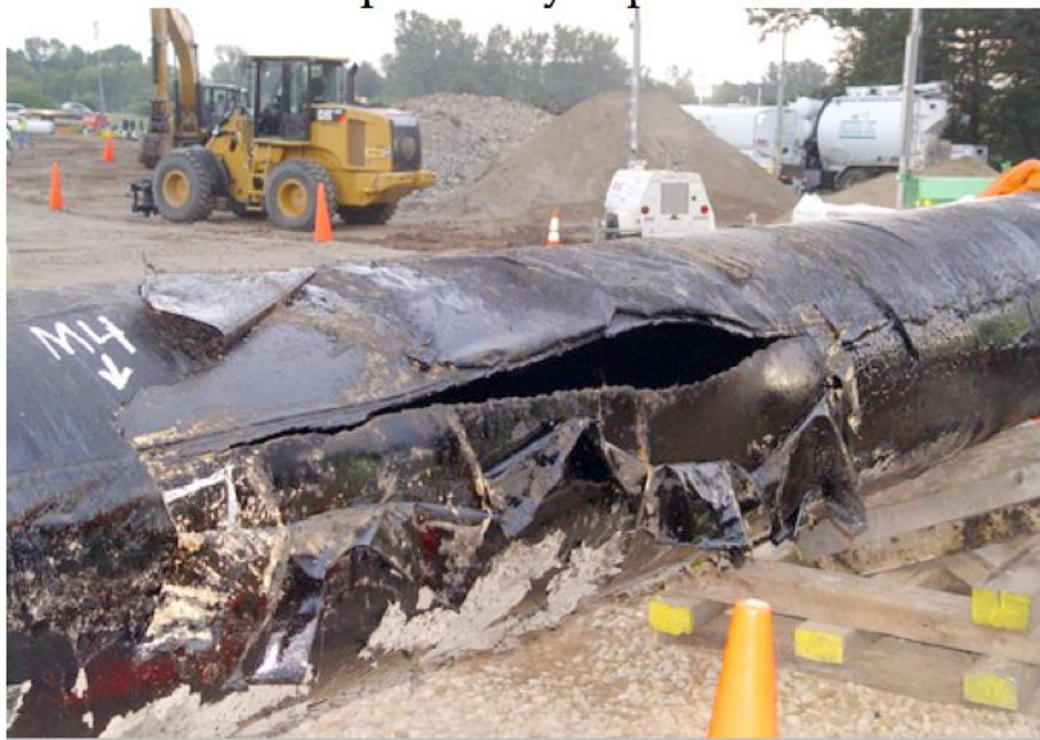
Figure 4 ERW Longitudinal Failure 15
