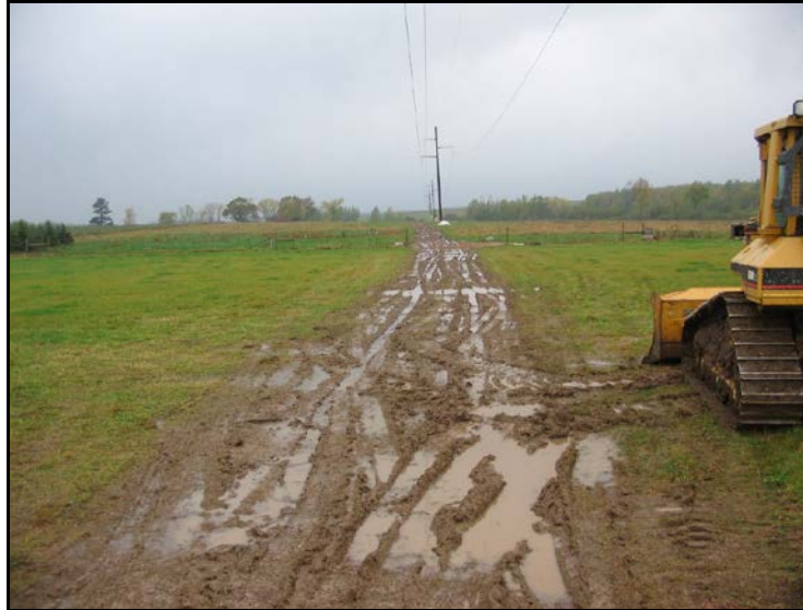
Figure 3 Rutting in Agricultural Lands
