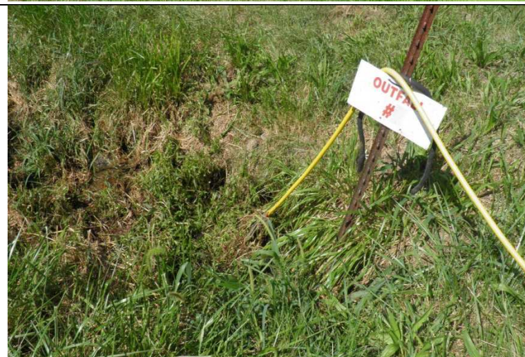
Photograph #: 6 Taken by: Michael Womack Entity: BCRSD - Highfield Acres Wastewater Treatment Facility Permit: #MO-0053376 Location: Boone Description: Observation of Outfall #002 with the missing number 2. The hose was observed to be draped over the sign but was not observed to be entering the lagoon. Date Taken: September 1, 2016 Program: WPC Unit
