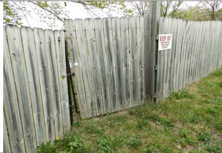
Photograph #: 1 Taken by: Michael Heaton Entity: BCRSD, Lee Heights Wastewater Treatment Facility Permit: #MO-0102113 Location: Boone County Description: Front entrance to the facility with a sign restricting access. Date Taken: May 2, 2018 Program: WPC Unit
