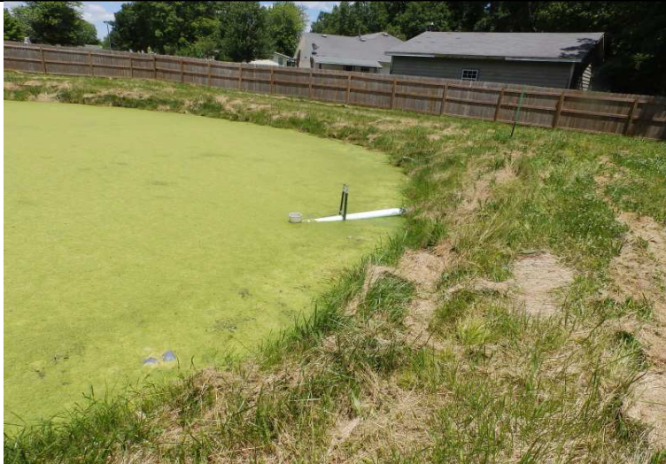
Photograph #: 4 Taken by: Leland Maize Entity: BCSD, Cedar Gate Subdivision Permit: #MO-0096415 Location: Boone County Description: Inlet side of the discharge pipe. A T fitting was in place on the inlet side. Date Taken: June 7, 2016 Program: WPC Unit
