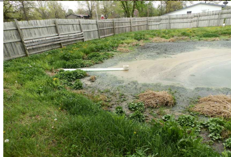
Photograph #: 3 Taken by: Michael Heaton Entity: BCRSD, Lee Heights Wastewater Treatment Facility Permit: #MO-0102113 Location: Boone County Description: View of the discharge pipe in the lagoon. Sludge accumulation is visible around the bank. Date Taken: May 2, 2018 Program: WPC Unit
