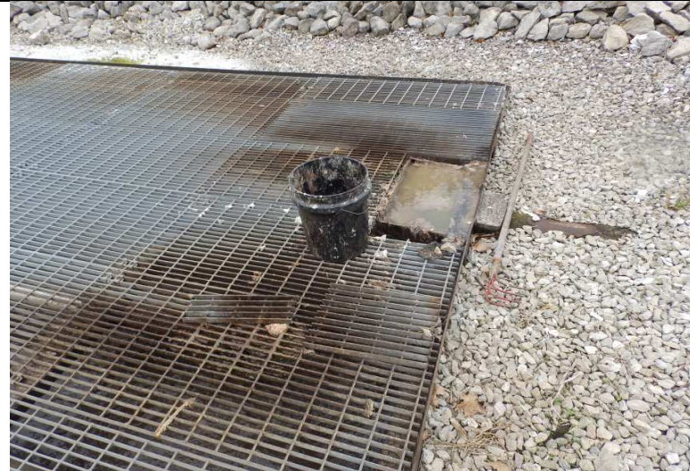
Photograph #: 8 Taken by: Michael Heaton Entity: BCRSD, Oberlin Valley Wastewater Treatment Facility Permit: #MO-0117323 Location: Boone County Description: View of bar screen at the facility. Program: WPC Unit
