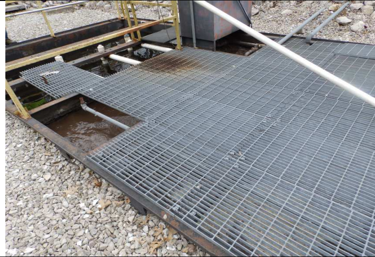
Photograph #: 7 Taken by: Michael Heaton Entity: BCRSD, Oberlin Valley Wastewater Treatment Facility Permit: #MO-0117323 Location: Boone County Description: Extended aeration facility. Date Taken: May 2, 2018 Program: WPC Unit
