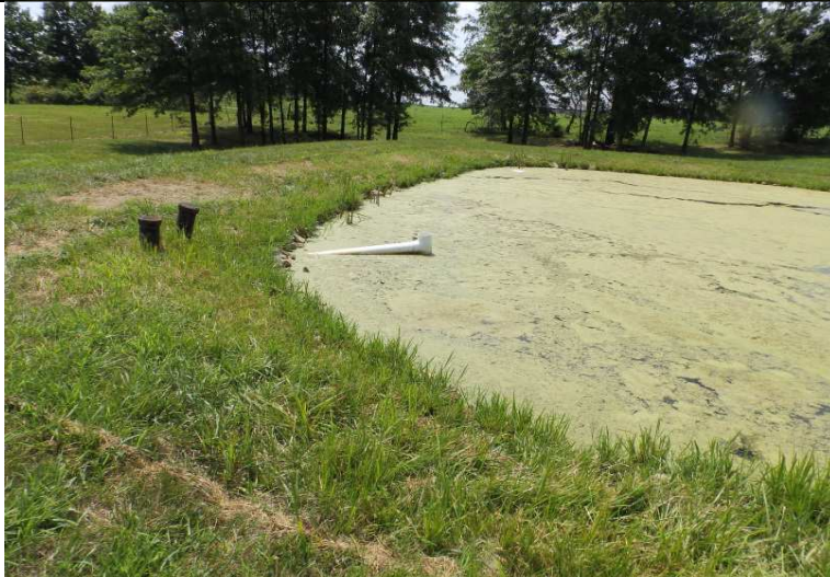
Photograph #: 5 Taken by: Leland Maize Entity: BCRSD, Quarter Mile Hills Subdivision Permit: #MO-0126446 Location: Boone County Description: Inlet side of the discharge pipe with a T-fitting on the end. Date Taken: July 27, 2016 Program: WPC Unit
