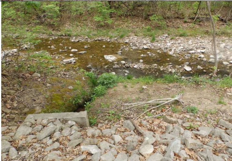
Photograph #: 3 Taken by: Michael Heaton Entity: BCRSD, Oberlin Valley Wastewater Treatment Facility Permit: #MO-0117323 Location: Boone County Description: View of the outfall location. Sludge and algae was observed in the stream below the outfall. Date Taken: May 2, 2018 Program: WPC Unit
