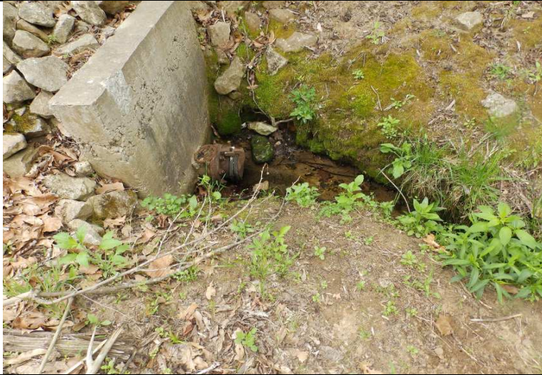
Photograph #: 4 Taken by: Michael Heaton Entity: BCRSD, Oberlin Valley Wastewater Treatment Facility Permit: #MO-0117323 Location: Boone County Description: Outfall #001 Date Taken: May 2, 2018 Program: WPC Unit
