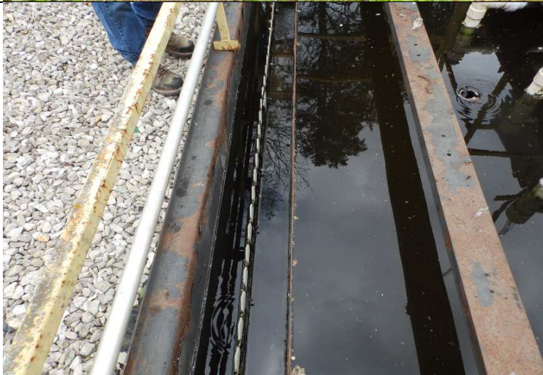
Photograph #: 6 Taken by: Michael Heaton Entity: BCRSD, Oberlin Valley Wastewater Treatment Facility Permit: #MO-0117323 Location: Boone County Description: Clarifier weir. Date Taken: May 2, 2018 Program: WPC Unit
