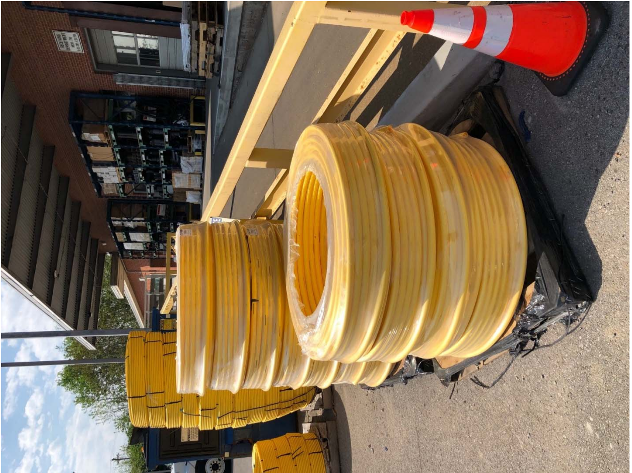
Figure 20, Spire East, Plastic Pipe
