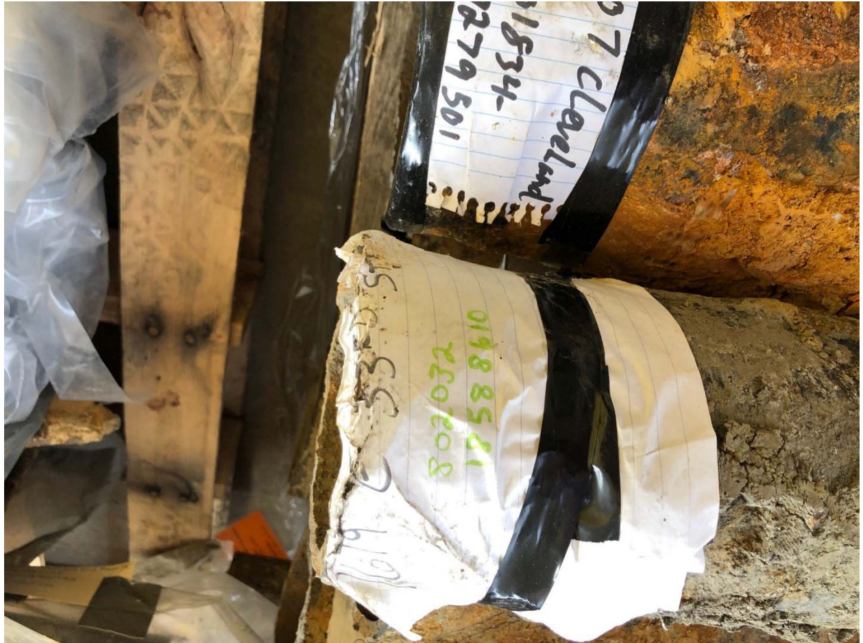
Figure 28, Spire East, Cast Iron, Work Order #18588610
