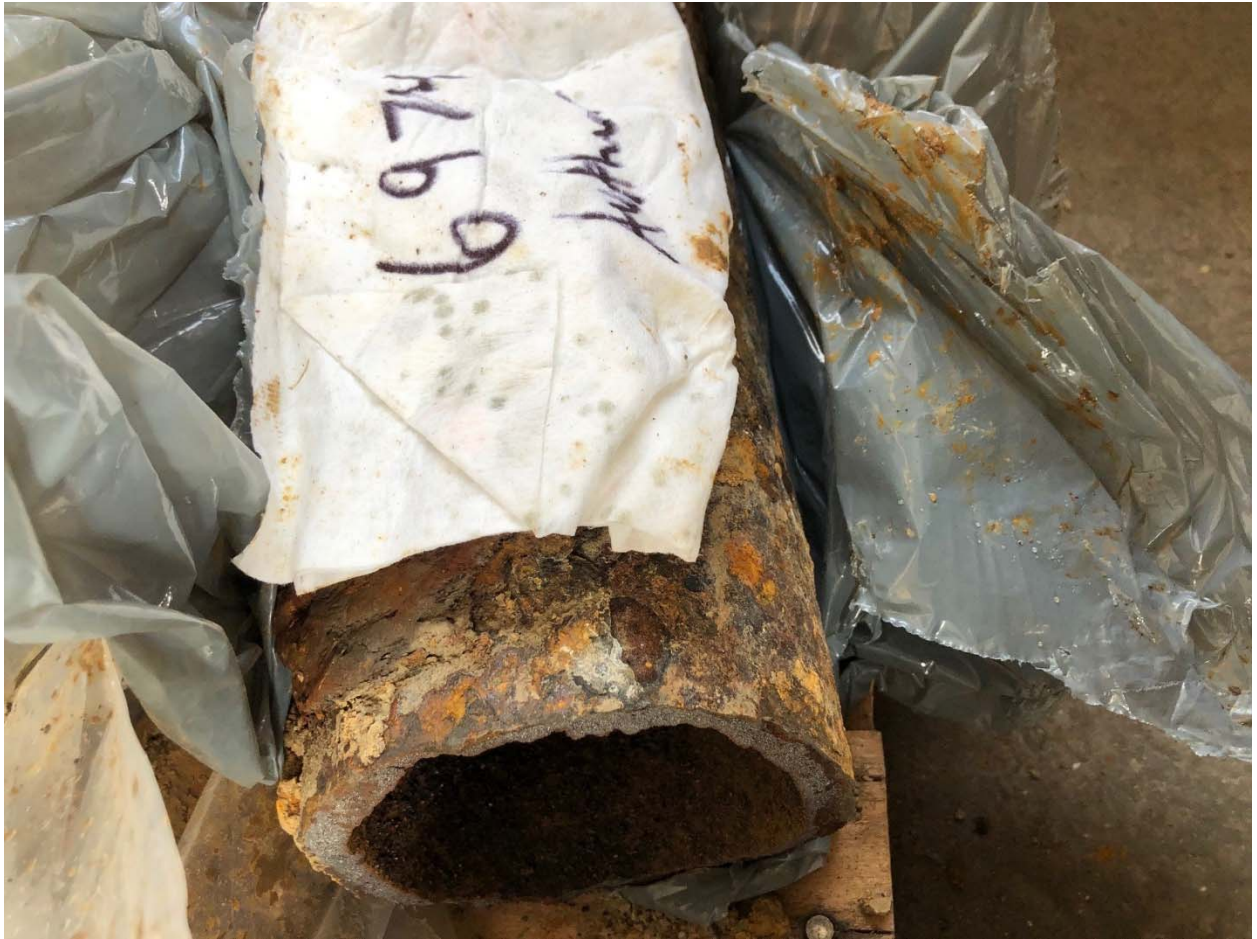
Figure 41, Spire West, Cast Iron
