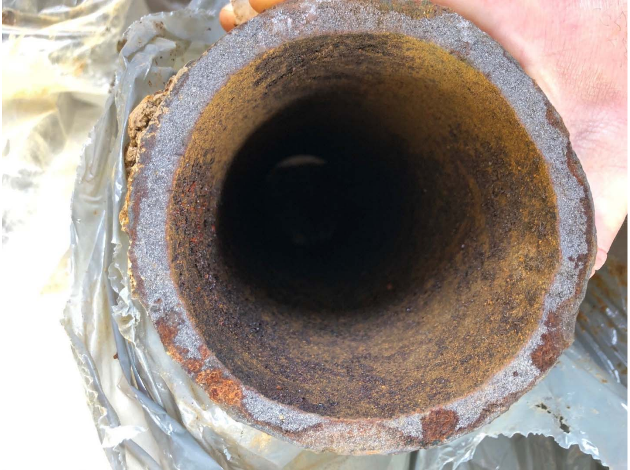
Figure 43, Spire West, Cast Iron
