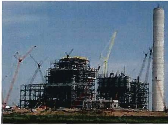
Power plant construction in late summer 2009 at the Prairie State Energy Campus. - Provided/BND
