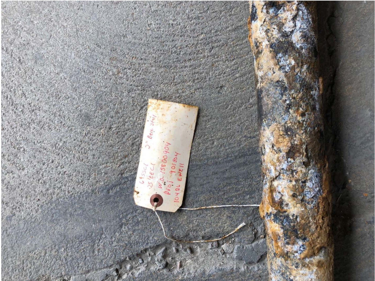
Figure 37, Spire West, Bare Steel, Work Order #15800904
