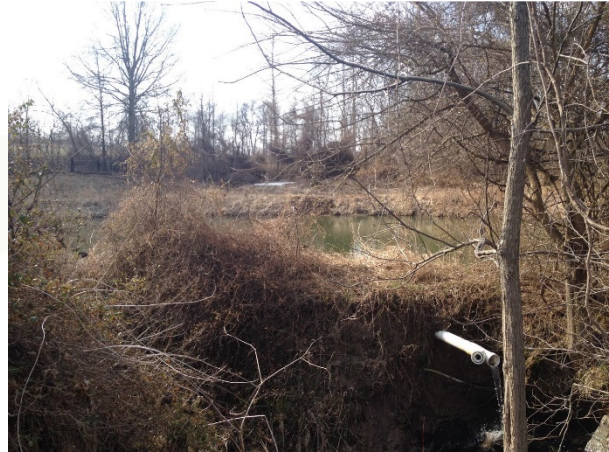
Old Lagoon with Illegal Untreated Drain
