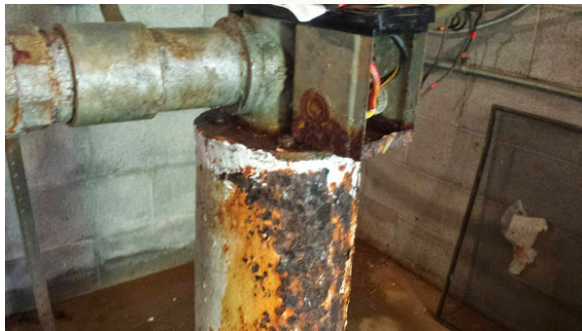
Corroded Hillcrest Drinking Water Well Head
