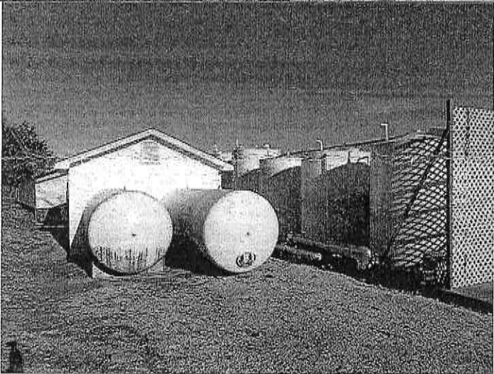
PHOTOGRAPH #6 TAKEN BY: Darrell Barber ENTITY: Camden County PWSD #5 - Clearwater Condos PERMIT: MO3302557 LOCATION: Outside of well house DESCRIPTION: Two hydropneumatic pressure tanks, five ground storage tanks and well house. DATE TAKEN: December 18, 2018 PROGRAM: Public Drinking Water Branch
