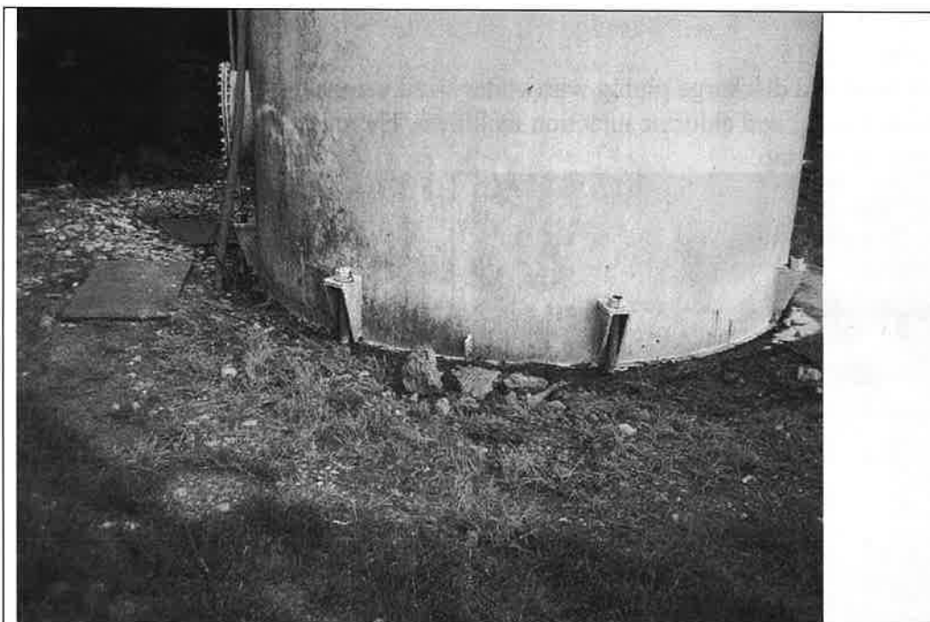
Location: Seven Trails West Photographer: Michael Grose Photograph Date: May 7, 2015 Comments: Tank base with dirt and standing water in contact with the tank base causing aggravated corrosion around the tank base.
