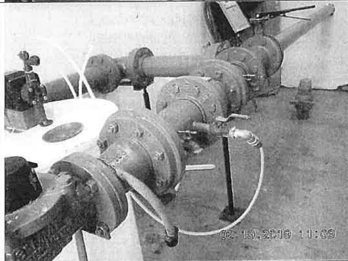
PHOTOGRAPH #2 TAKEN BY: Johnny O'Dell ENTITY: Lakeside at Cross Creek PERMIT: MO5031496 LOCATION: Inside wellhouse DESCRIPTION: Chlorine injection point DATE TAKEN: February 19, 2019 PROGRAM: Public Drinking Water Branch
