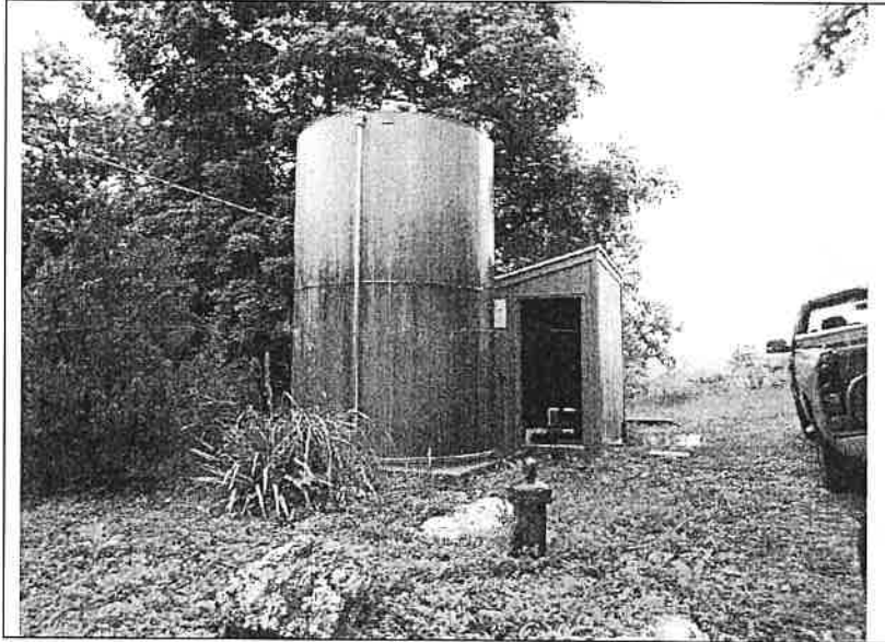
Location: Makalu Estates Photographer: Darrell Barber Photograph Date: May 20, 2015 Comments: Well #2, well house and 3,500-gallon ground storage tank.
