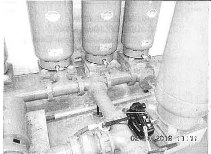
PHOTOGRAPH #5 TAKEN BY: Johnny O'Dell ENTITY: Lakeside at Cross Creek PERMIT: MO5031496 LOCATION: Inside wellhouse DESCRIPTION: Bladder tanks DATE TAKEN: February 19, 2019 PROGRAM: Public Drinking Water Branch
