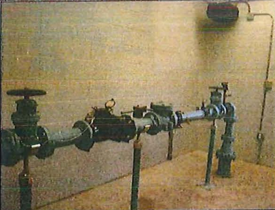
Photo #:002 Date Taken: 10/26/2016 By: Michelle Oglesby Program: PDWB File: Crawford County Location: Indian Hills Utilities Operating Co. Inc. Description: Well #1 - Piping
