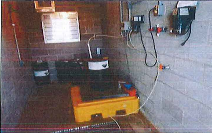
Photo #: 005 Date Taken: 01/24/2018 By: Michael Wyatt Program: PDWB File: Hillcrest Utility Operating Co., Inc. – General Location: Chlorine feed room Description: Chlorine feed system.
