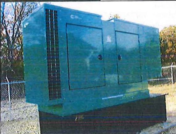
Photo #:008 Date Taken: 10/26/2016 By: Michelle Oglesby Program: PDWB File: Crawford County Location: Indian Hills Utilities Operating Co. Inc. Description: Well #1 – Generator
