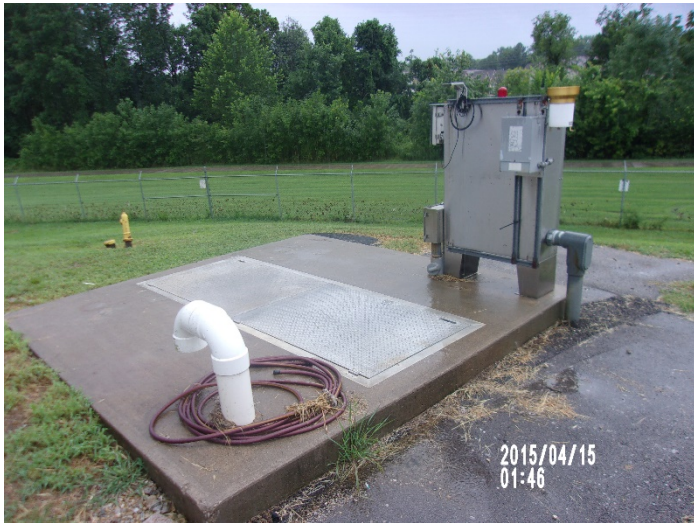
Photograph: # 1. Taken By: Oscar Vazquez Date Taken: July 29, 2019 Program: ECA Unit Entity: Eureka WWTF Permit: MO-0039569 Location: Influent Lift Station Description: Wet well and pump control panel.
