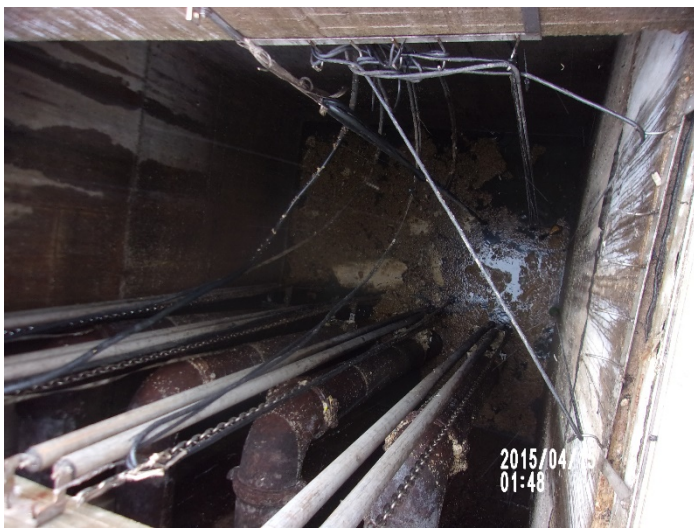
Photograph: # 2. Taken By: Oscar Vazquez Date Taken: July 29, 2019 Program: ECA Unit Entity: Eureka WWTF Permit: MO-0039569 Location: Influent Lift Station Description: Wet well with four pump discharge lines.
