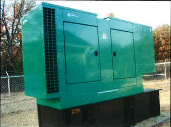
Photo #:008 Date Taken: 10/26/2016 By: Michelle Oglesby Program: PDWB File: Crawford County Location: Indian Hills Utilities Operating Co. Inc. Description: Well #1 – Generator
