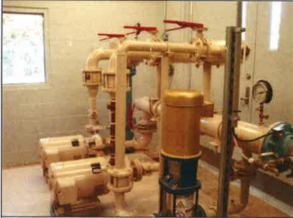
Photo #:006 Date Taken: 10/26/2016 By: Michelle Oglesby Program: PDWB File: Crawford County Location: Indian Hills Utilities Operating Co. Inc. Description: Well #1 – Booster Pump Station
