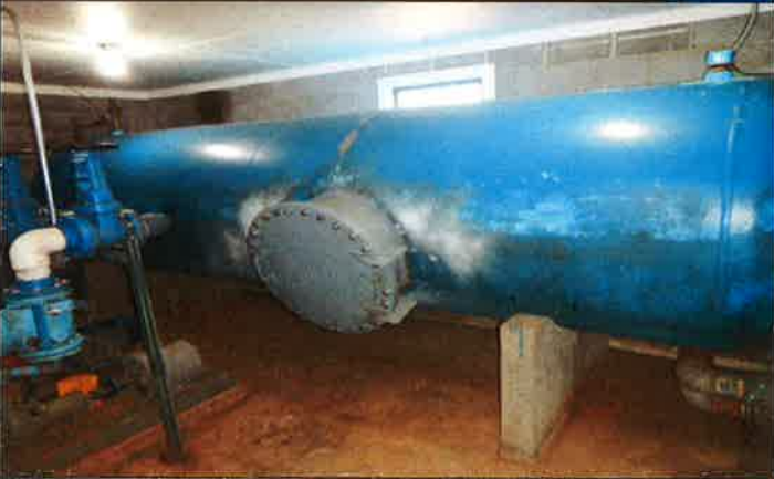
Photo #: 003 Date Taken: 01/24/2018 By: Michael Wyatt Program: PDWB File: Hillcrest Utility Operating Co., Inc. – General Location: Well house Description: ~2,100 gallon hydro-pneumatic pressure tank.
