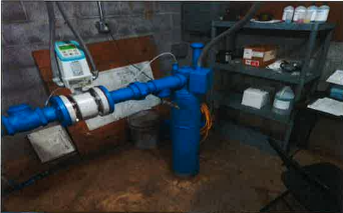
Photo #: 001 Date Taken: 01/24/2018 By: Michael Wyatt Program: PDWB File: Hillcrest Utility Operating Co., Inc. – General Location: Well house Description: Well.
