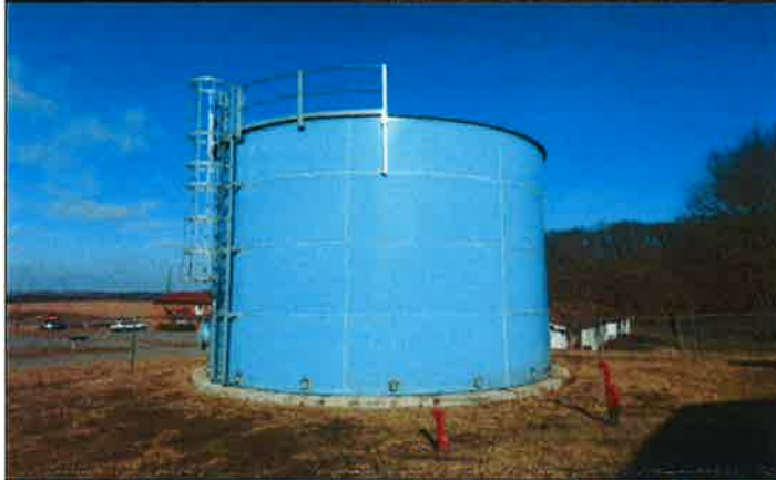
Photo #: 007 Date Taken: 01/24/2018 By: Michael Wyatt Program: PDWB File: Hillcrest Utility Operating Co., Inc. – General Location: Tank site Description: 58,000 gallon ground storage tank.
