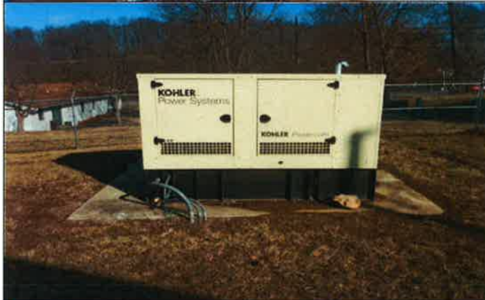
Photo #: 006 Date Taken: 01/24/2018 By: Michael Wyatt Program: PDWB File: Hillcrest Utility Operating Co., Inc. – General Location: Back of well house building Description: Stationary generator.
