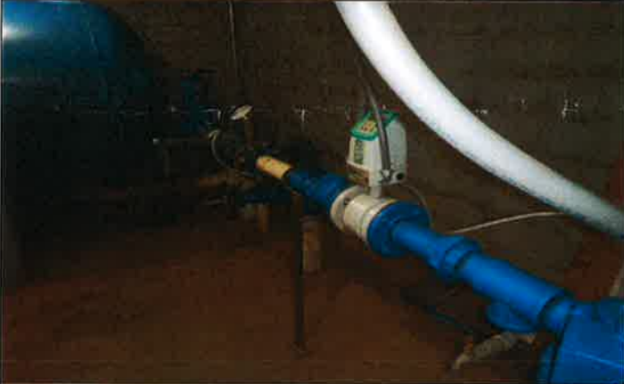
Photo #: 002 Date Taken: 01/24/2018 By: Michael Wyatt Program: PDWB File: Hillcrest Utility Operating Co., Inc. – General Location: Well house Description: Discharge piping.
