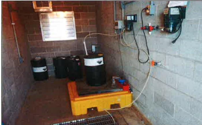
Photo #: 005 Date Taken: 01/24/2018 By: Michael Wyatt Program: PDWB File: Hillcrest Utility Operating Co., Inc. – General Location: Chlorine feed room Description: Chlorine feed system.
