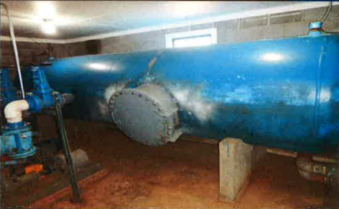
Photo #: 003 Date Taken: 01/24/2018 By: Michael Wyatt Program: PDWB File: Hillcrest Utility Operating Co., Inc. – General Location: Well house Description: ~2,100 gallon hydro-pneumatic pressure tank.
