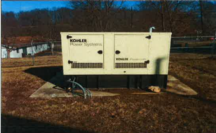
Photo #: 006 Date Taken: 01/24/2018 By: Michael Wyatt Program: PDWB File: Hillcrest Utility Operating Co., Inc. – General Location: Back of well house building Description: Stationary generator.
