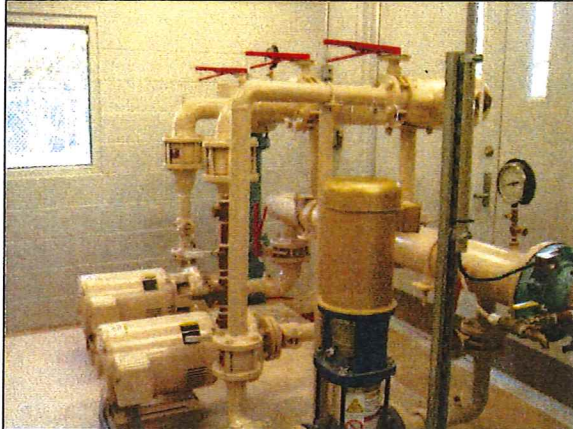
Photo #:006 Date Taken: 10/26/2016 By: Michelle Oglesby Program: PDWB File: Crawford County Location: Indian Hills Utilities Operating Co. Inc. Description: Well #1 – Booster Pump Station
