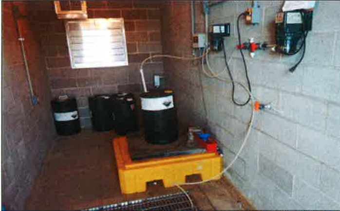
Photo #: 005 Date Taken: 01/24/2018 By: Michael Wyatt Program: PDWB File: Hillcrest Utility Operating Co., Inc. – General Location: Chlorine feed room Description: Chlorine feed system.
