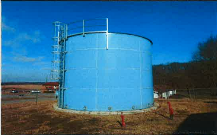
Photo #: 007 Date Taken: 01/24/2018 By: Michael Wyatt Program: PDWB File: Hillcrest Utility Operating Co., Inc. – General Location: Tank site Description: 58,000 gallon ground storage tank.
