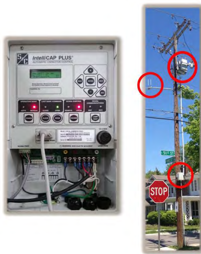
Figure 2-63: Typical Capacitor Bank Installation
