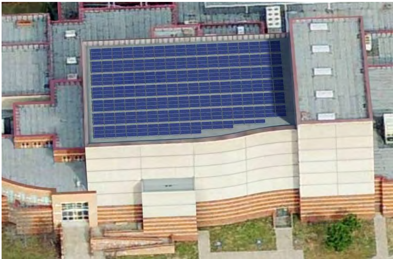
Figure 1-28: Paseo High School Rooftop Solar PV System
