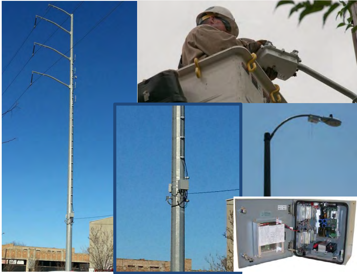
Figure 2-21 Installed AMI FAN Infrastructure
