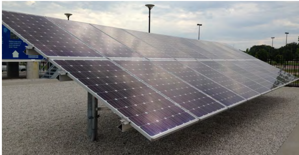
Figure 3-28: 5 kW Photovoltaic Array at SmartGrid Innovation Park
