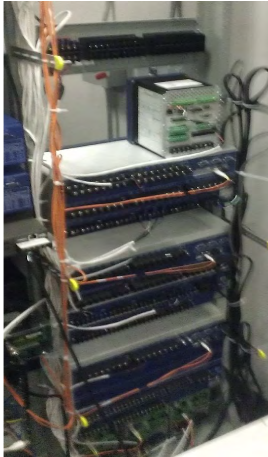
Figure 2-47: GOOSE Lab Testing Rack Setup
