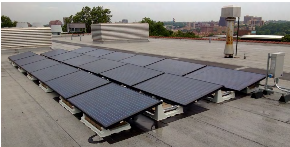
Figure 2-75: Typical Commercial PV Installation
