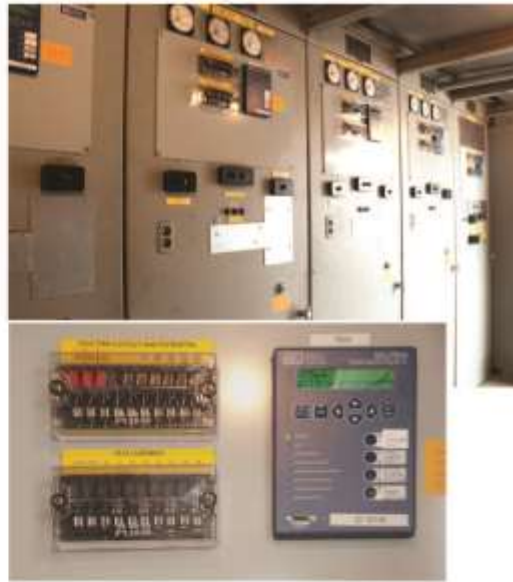
Older electro-mechanical substation relays replaced with new digital IEC-61850 compatible relays by SEL
