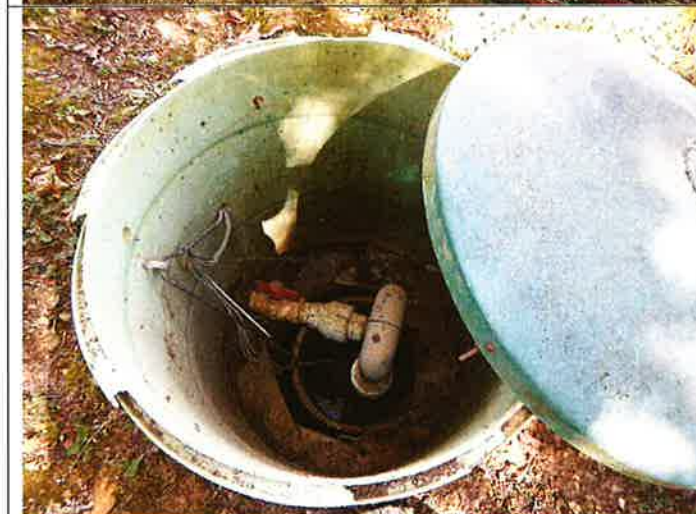
Photograph #: 012 Taken by: Elizabeth Stephens Entity: Confluence Rivers-Port Perry WWTF Permit: MOG823126 Location: Perry County Description: Inside view of lift station. Date Taken: October 1, 2020 Program: WPC Unit
