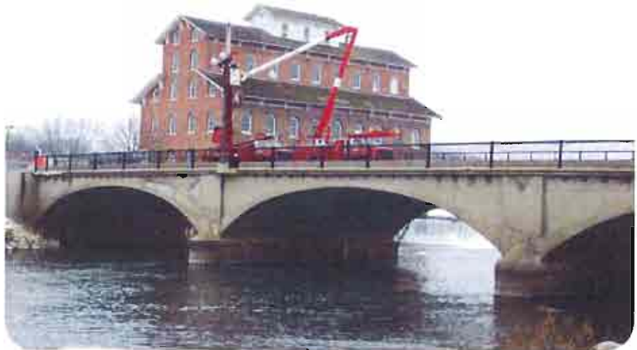
New light fixtures on the bridge near the Wapsipinicon Mill are installed.
