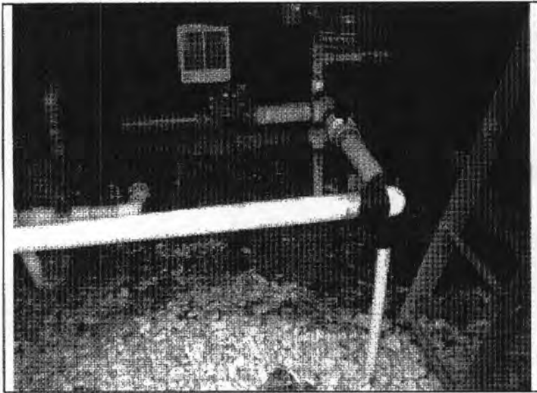
Location: Taney Co Water LLC – Venice Photographer: Katie Hirtz Photograph Date: December 10, 2014 Comments: Bladder tank and booster pump serving uphill connections at Red Rock.
