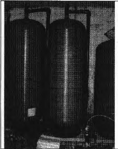
Location: Taney Co Water LLC – Venice Photographer: Katie Hirtz Photograph Date: December 10, 2014 Comments: Bladder tank and chlorine detention tanks at Honey Lane.
