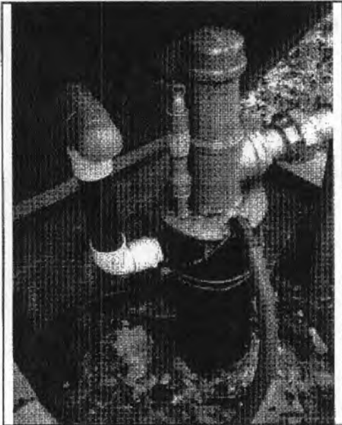
Location: Taney Co Water LLC – Venice Photographer: Katie Hirtz Photograph Date: December 10, 2014 Comments: Red Rock well. The department recommends securing the access hatch.
