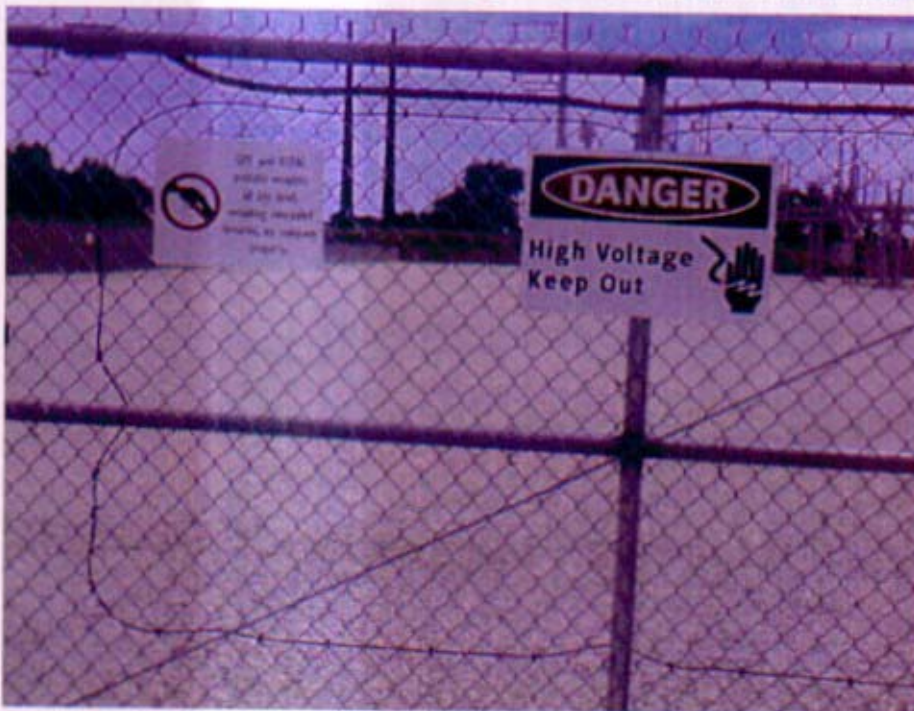
Photo No. 5-6: Weapons Prohibition and Danger/High Voltage Signs on Substation Perimeter Fence Gate. The "Danger" sign is mounted approx. every fifty feet on the perimeter fence.
