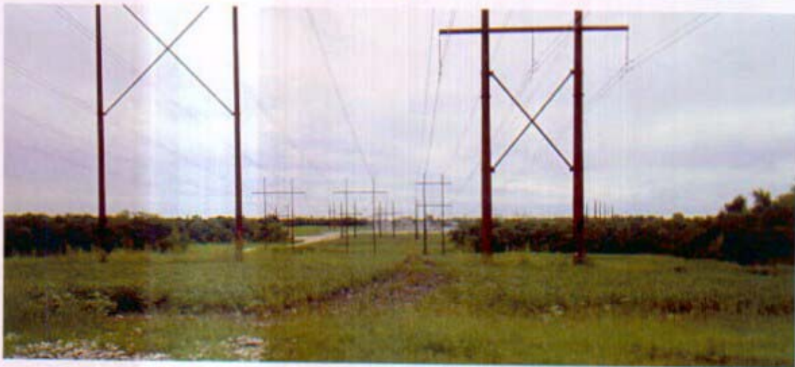
Photo No. 3 – View from the site boundary (property line) looking south from within the existing transmission line easement from 203 rd St.
