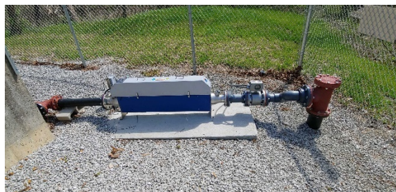
UV disinfection system
