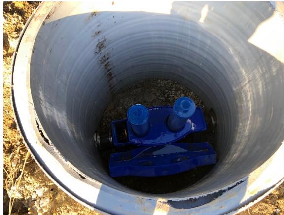
New chlorine disinfection equipment
