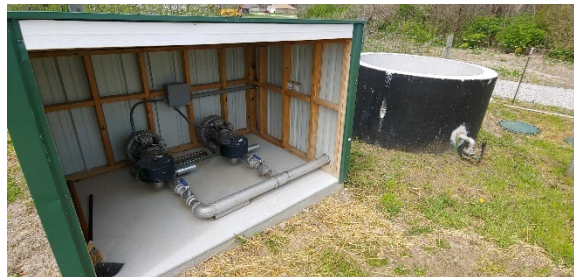
15 16 New blowers and MBBR unit
