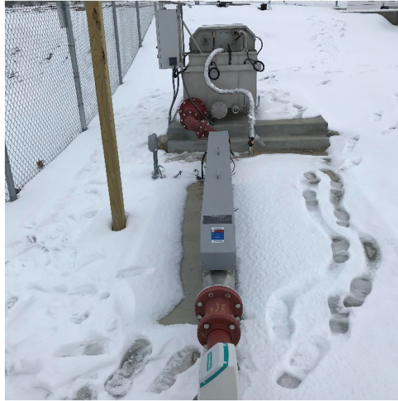
UV Disinfection system
