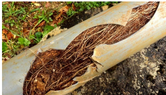
7 8 Example of vitrified clay pipe damaged by root infiltration allowing I&I flows
