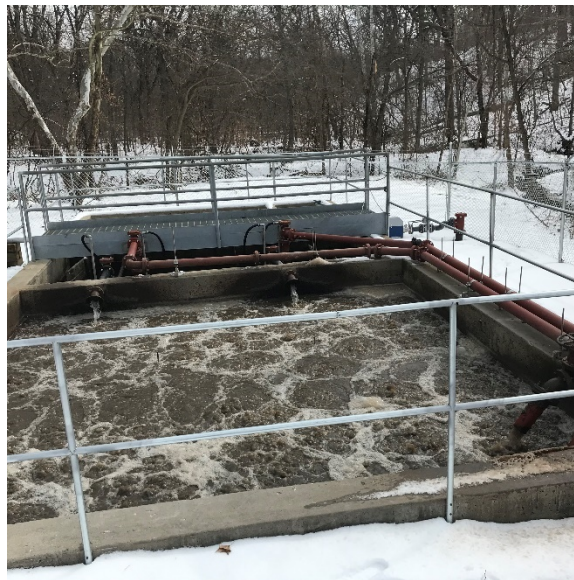
Aeration basin post upgrade
