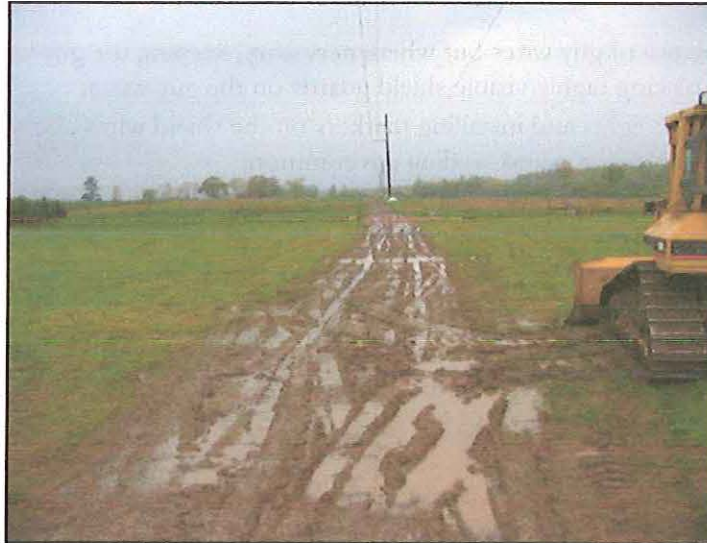
Figure 3 Rutting in Agricultural Lands
