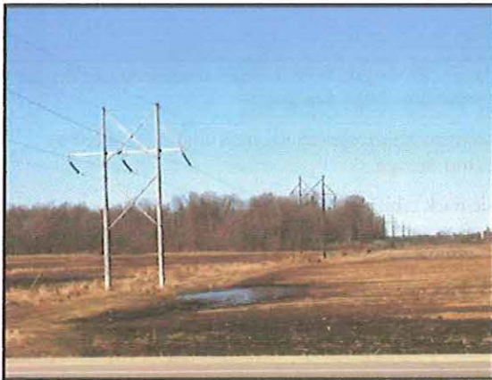
Figure 1 Typical Two-Pole, H-frame Structure
