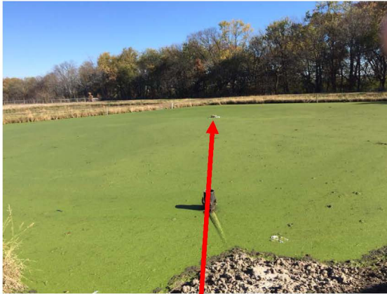
2 nd Lagoon Cell With Failed Aerator
