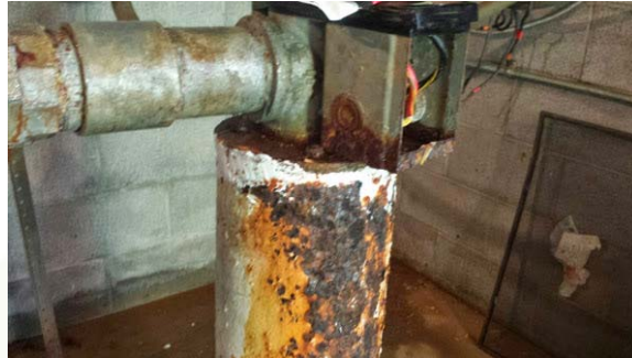
Corroded Hillcrest Drinking Water Well Head
