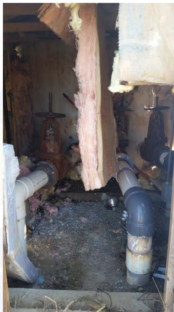
Looking Down Roof Hole over Water System Connections to the original Water Tower
