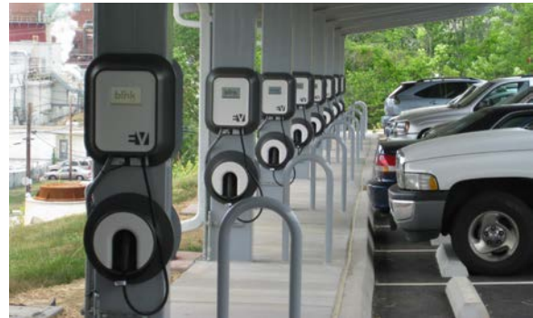
Photo 1. This series of Level 2 EVSE were installed by the EV Project. Photo from INL.
