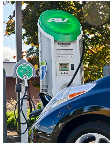
Photo 13. One of many side by side DCFC and Level 2 EVSE installed along the West Coast Electric Highway in Oregon and Washington. Photo from Washington State Department of Transportation (WSDOT).
