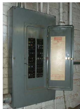
Photo 21. Electrical panel. Photo from NYSERDA.
