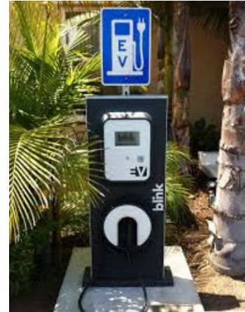
Photo 15. The connector on this EVSE unit is low to the ground to meet ADA accessibility requirements. Photo from Ecotality.
