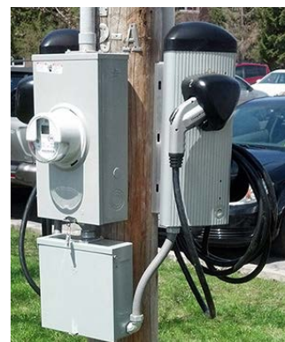
Photo 20. An electrical meter mounted alongside the EVSE and connected with conduit. Photo from NYSERDA.
