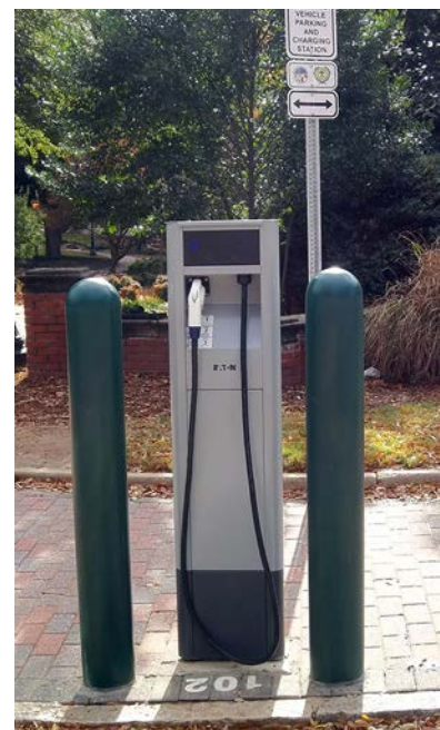
Photo 2. Pedestal-mounted EVSE installed by the City of Raleigh, N.C., for free public use. Photo from Kathy Boyer, NREL 18520
