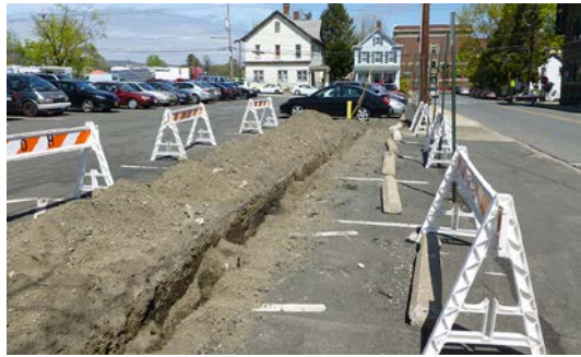
Photo 7. Trenching through a parking lot to install a public dual-port Level 2 EVSE in Haverstraw, N.Y. Photo from New York State Research and Development Authority (NYSERDA).
