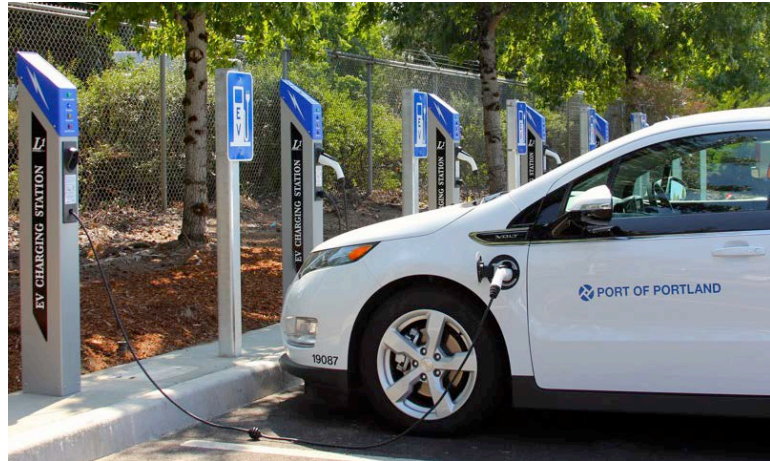
Photo 6. Portland International Airport installed 42 Level 1 EVSE for employees and airport customers. Photo from Telefonix.
