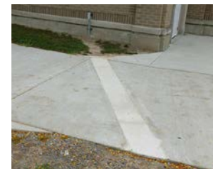
Photo 8. Trenching through soil and sidewalk was needed to install EVSE at the University of Buffalo. Photo from NYSERDA.
