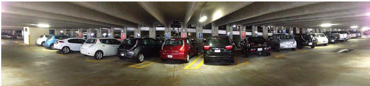
Photo 16. Electrical outlets are available along a row of parking stalls for PEV drivers to charge their vehicles using a Level 1 cordset. Photo from Jonathan Kirchner, Coca-Cola.
