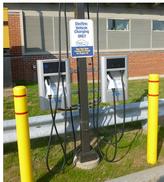
Photo 17. These two EVSE are located close to the building, reducing trenching costs. Photo from NYSERDA.
