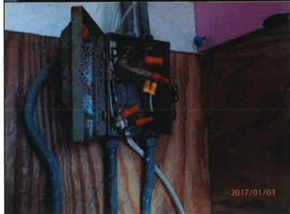
Photo #: 6 Date/Time Taken: 01/03/2017 at approx. 0918 hours By: Richard Morrow Program: PDW Unit File: 3.200 Facility: Kuhle H20 Location: Well House Description: The well house does not meet the minimum sanitary construction standards. Some of the wiring is not in conduit and exposed, which is a safety issue.
