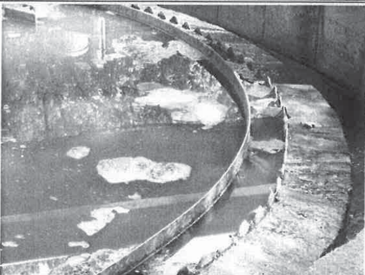
Photograph: #005 Taken By: Christopher Maher Facility: Villa Ridge Estates Permit: MO-0038237 Location: Secondary Clarifier
