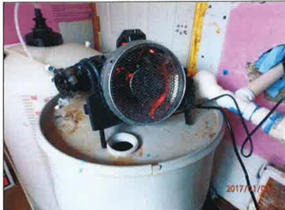
Photo #: 4 Date/Time Taken: 01/03/2017 at approx. 0916 hours By: Richard Morrow Program: PDW Unit File: 3.200 Facility: Kuhle H20 Location: Well House Description: The hypochlorite tank is not vented to the outside. The chlorine tank needs to be vented to the outside to prevent further corrosion to the piping and metal works inside the well house.
