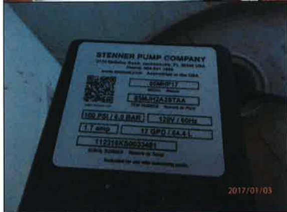
Photo #: 5 Date/Time Taken: 01/03/2017 at approx. 0916 hours By: Richard Morrow Program: PDW Unit File: 3.200 Facility: Kuhle H20 Location: Well House Description: There is only one operating chlorination pump. The system should maintain disinfection redundancy by having two pumps available in case the lead pump becomes inoperable.
