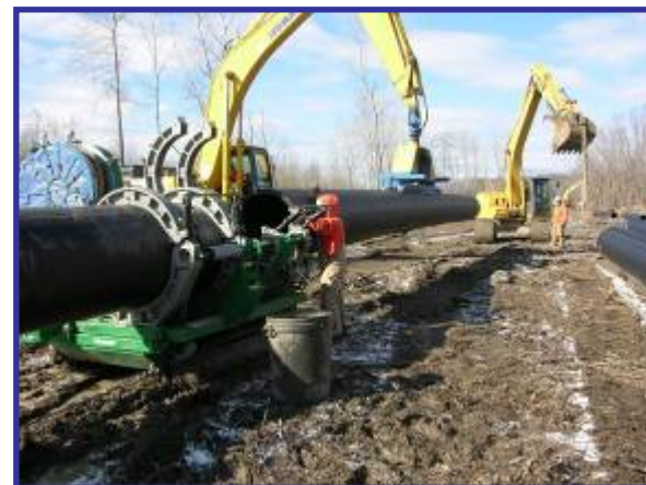
New Discharge Pipe
