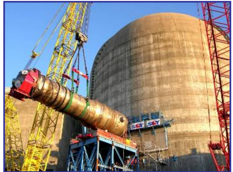
New Steam Generator
