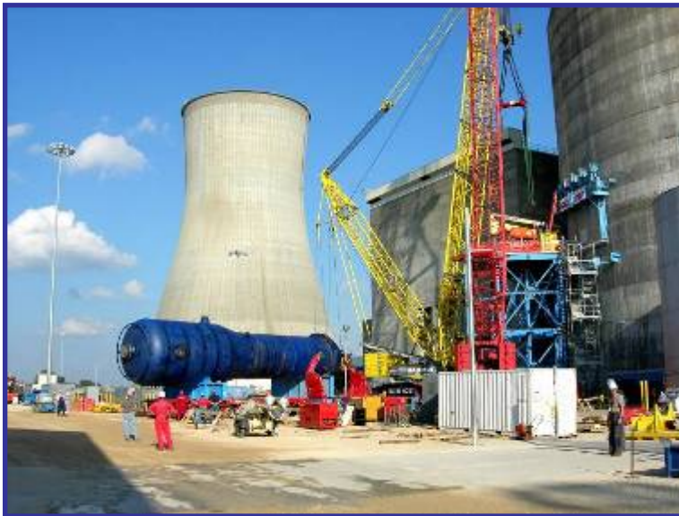
Old Steam Generator
