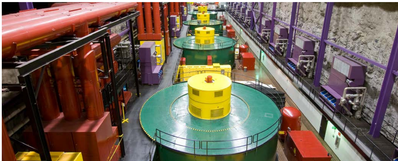
Figure 17-3 — Typical Hydroelectric Power Turbine Hall
