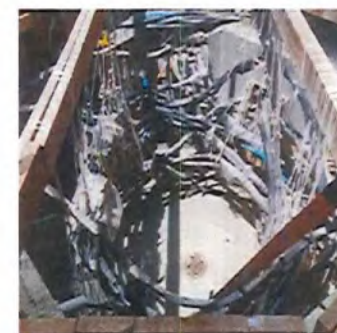
Highly congested manhole on 7 th St.
