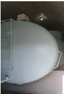
Mo Utilities Tank (Exterior)
