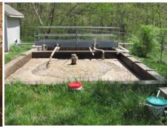
State Park – No Aeration or Railing
