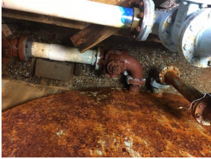
Indian Hills Storage Tank
