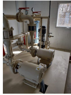
New Booster Pumps
