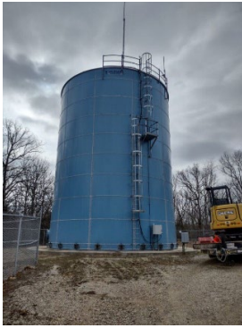
New Storage Tank
