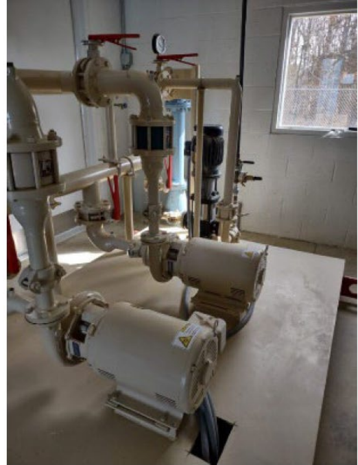
New Booster Pumps
