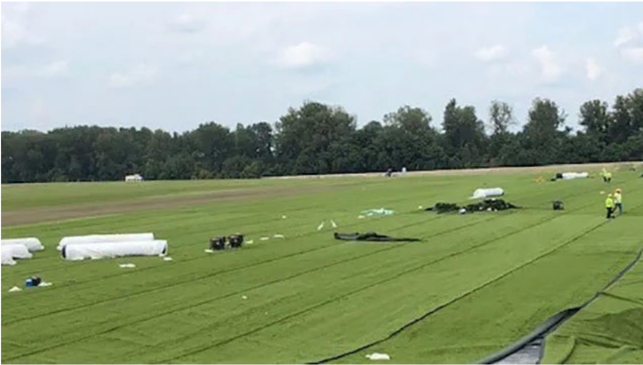
Crews finish covering the protective liner with turf and sand at Rush Island Energy Center. The cover is contoured for controlled rainwater drainage.
