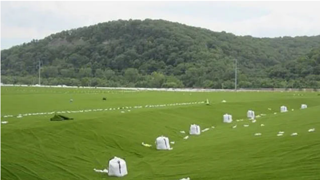
Weighted bags temporarily hold down the turf until sand is swept in, anchoring the turf to the liner below.
