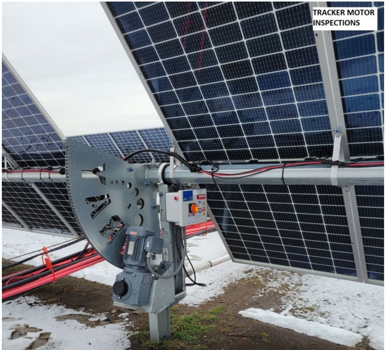
Tracker motor inspections
