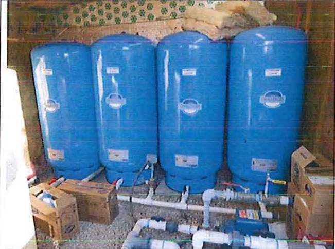
PHOTOGRAPH# 5 TAKEN BY: Darrell Barber ENTITY: Makalu Estates PERMIT: MO3031208 LOCATION: Inside well house DESCRIPTION: Four 119-gallon bladder tanks and related piping. DATE TAKEN: December 1, 2017 PROGRAM: Public Drinking Water Branch
