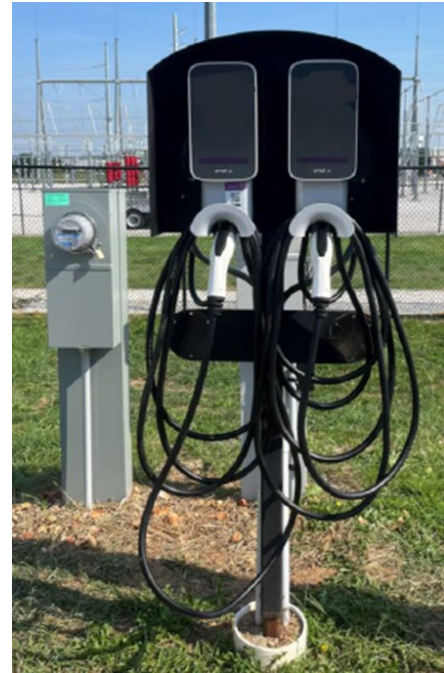
Figure 7: Home charger accuracy exploration installation at Liberty's operations center in Joplin
