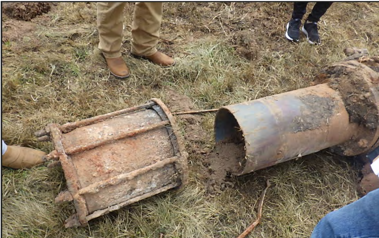
Figure 6: Photograph showing Dresser fitting previously installed on the North Leg of the Feeder line separated from the North Leg piping following the incident (Source: Staff Photograph July 19, 2023).
