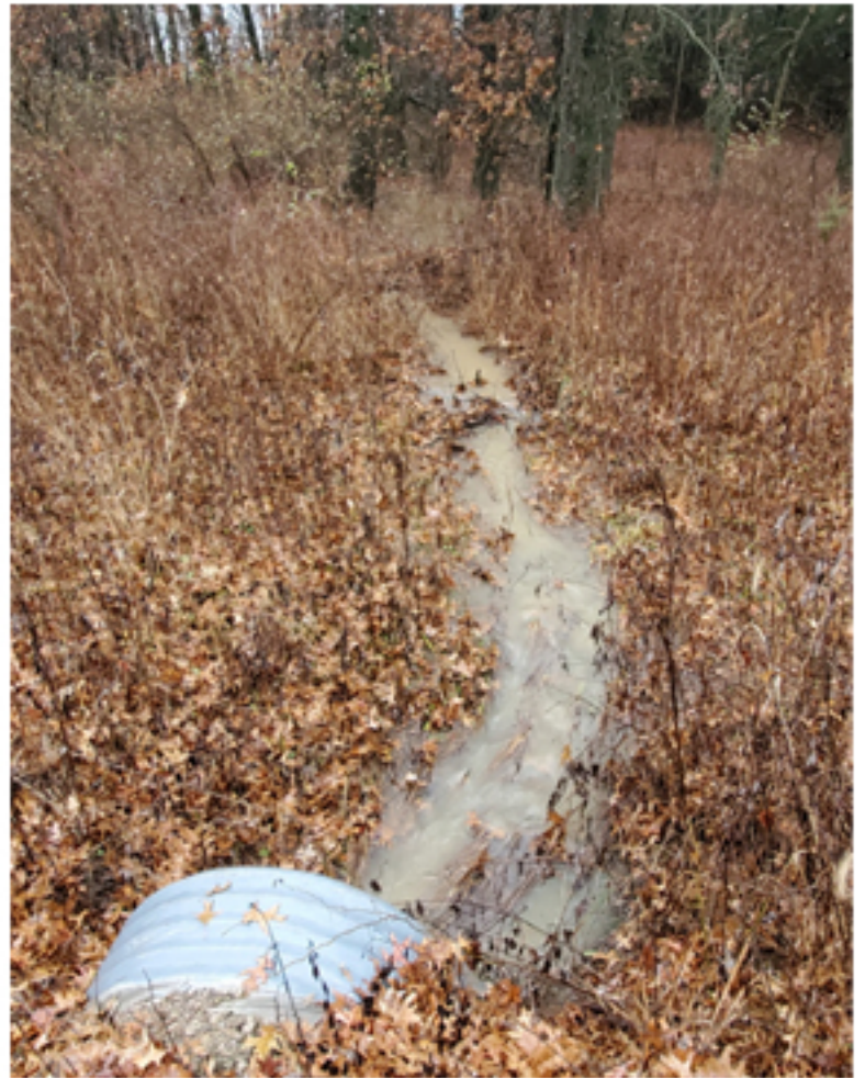
Water flowing from the east side of my land through the culvert under my drive, all downhill from where the easement will be.
