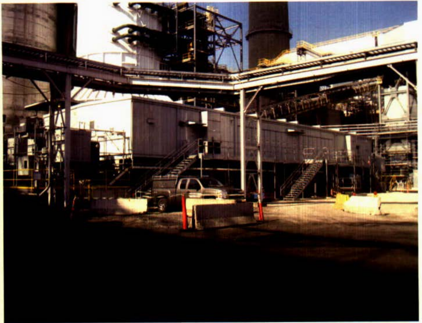
Another View of the Main PDC Building and Step-down Transformers
