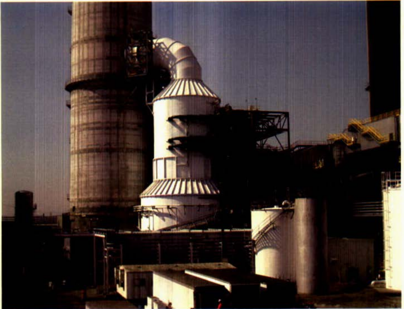
New Unit 1 Flue Gas Desulfurization System and Main Power Distribution Center (PDC) Building
