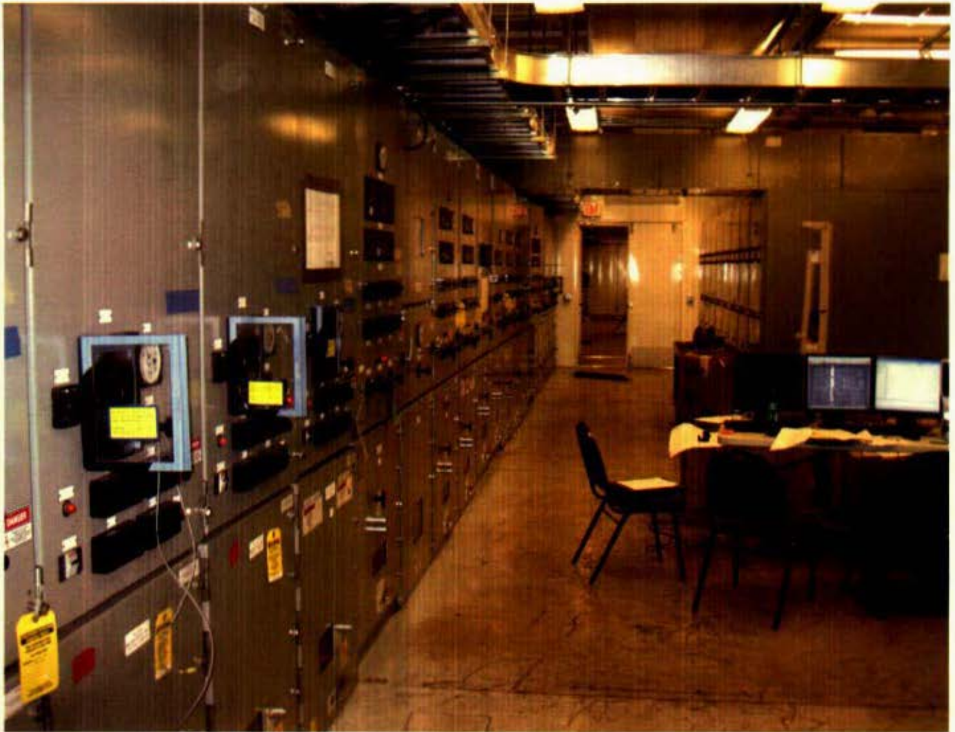
Some of the 4160V Breakers Inside the Main PDC Building
