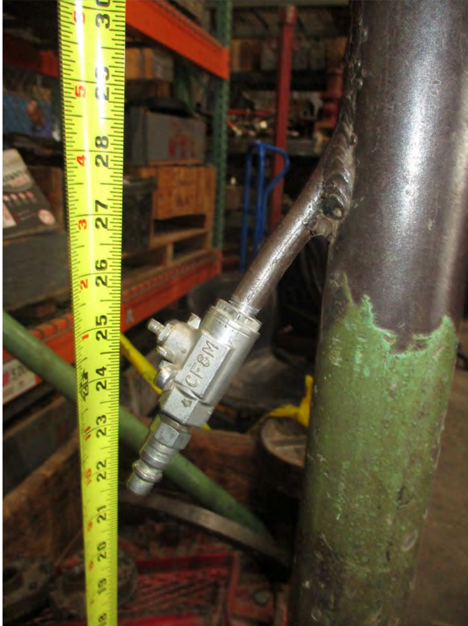
Figure 3 – Photograph of vent stack that was used at the incident location showing air hose connection for air handler, pipe extending diagonally into the vent stack with open end inside the vent stack, and valve used to allow the flow of air from a compressor into the vent stack. The venturi-effect of the air flowing upward and out of the vent stack to the atmosphere creates a vacuum from the vent stack below this location and from the pipe segment connected to the bottom of the vent stack. (Source: Staff Photograph)
