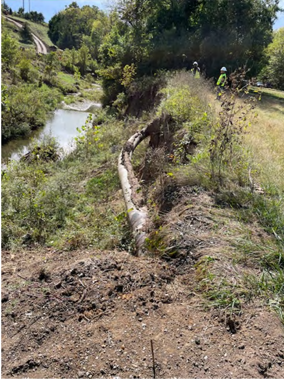
Figure 2 – Photograph showing Segment of Pipeline Exposed in Creek Bank (Source: Staff Photograph)
