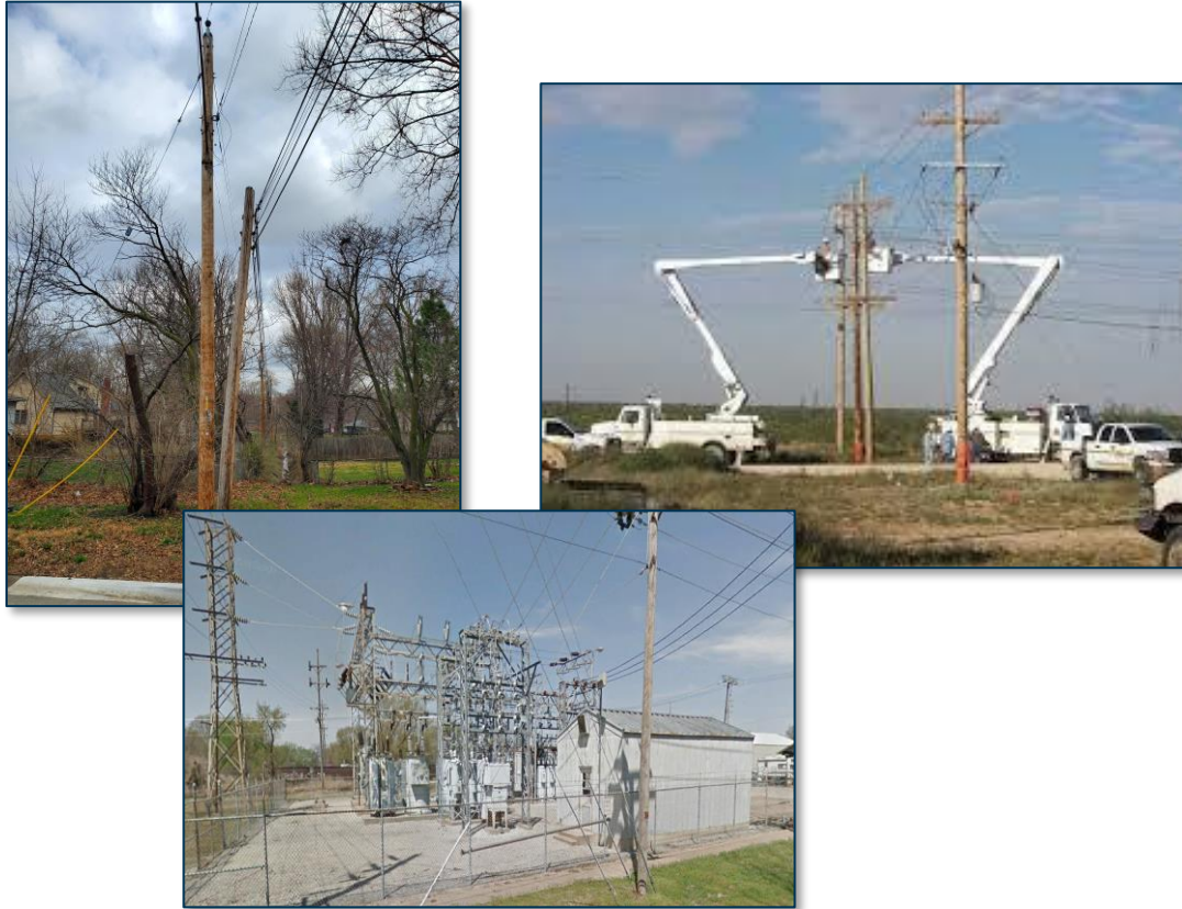
Rebuilding miles of aged overhead distribution lines and replacing aged substation assets to support customer reliability
